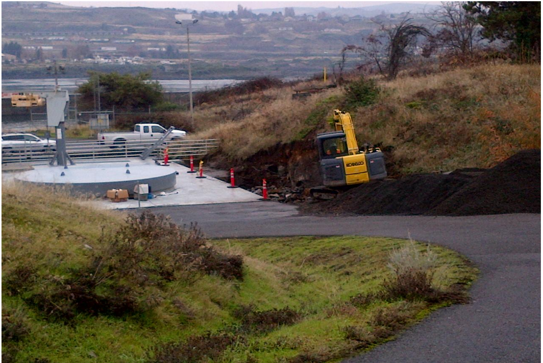
Wasco PUD excavating near their powerhouse to make space for transformer. Greater than 50' from north fishladder.
